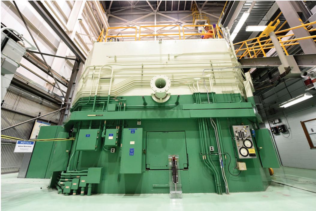
Figure 1. The Transient Reactor.
